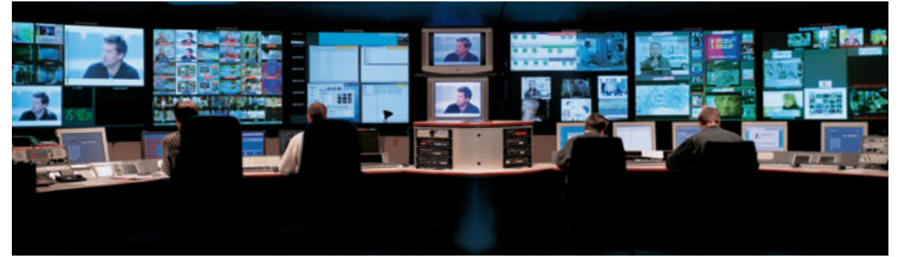
Canal+ Group's Digital Broadcasting Center in Paris
